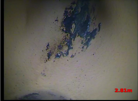
, 00:00:22, 2.81m Finish node type, major connection without manhole, reference number: Soil Vent
