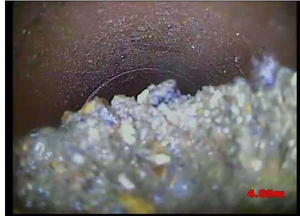
, 00:00:38, 4.09m Settled deposits, coarse, 80% cross-sectional area loss
